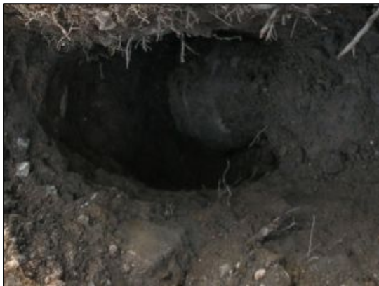
Figure 4. Detail of the gas pipe
