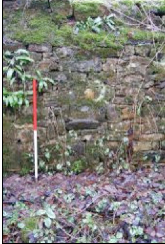
Figure 17. Blocked "window" in eastern elevation
