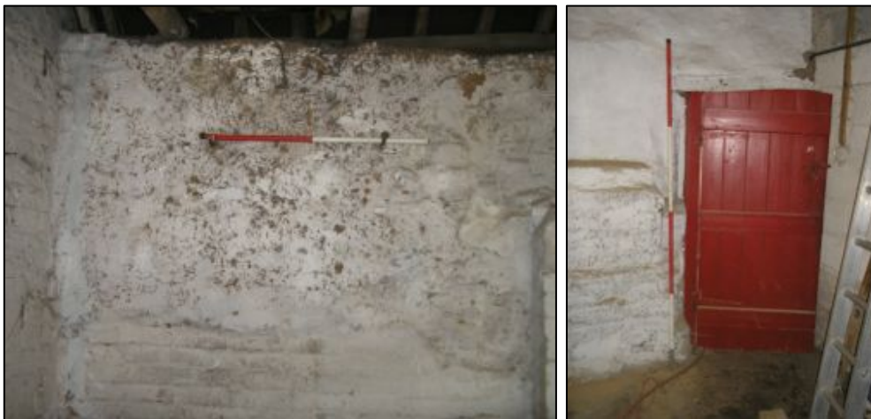
Figures 15 and 16. Detail of clay dabbin wall and modern door, north wall
